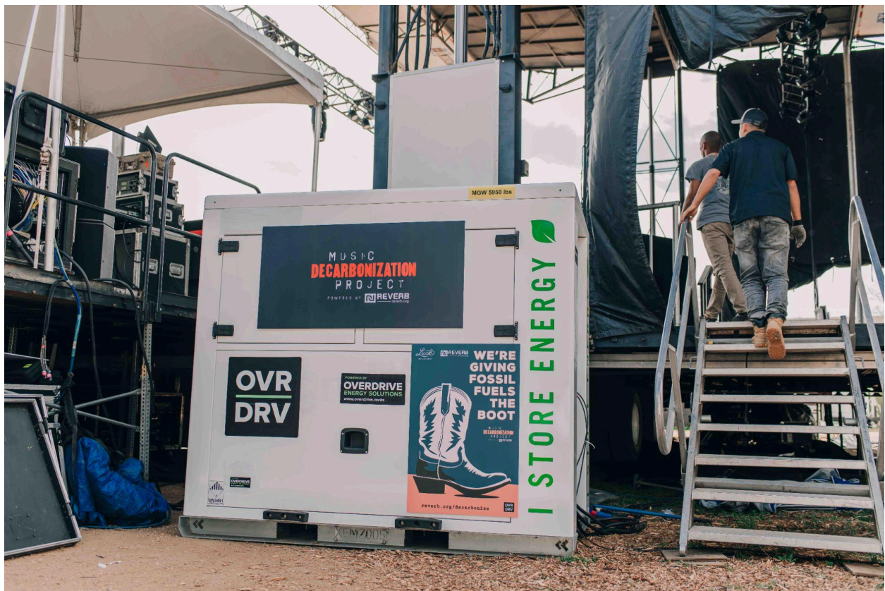
Luck Main Stage Battery
