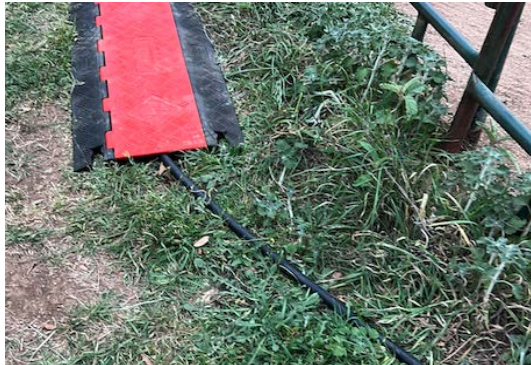
Image 5 - 10 Gauge DC Power Cables
