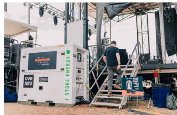
Image 7 - One of Two POWR2 Units at the WHQ Stage
